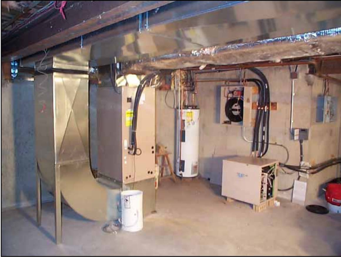
A 4-ton EarthLinked unit, air handler and heat exchanger for forced-air space heating and cooling, and domestic water heating.
