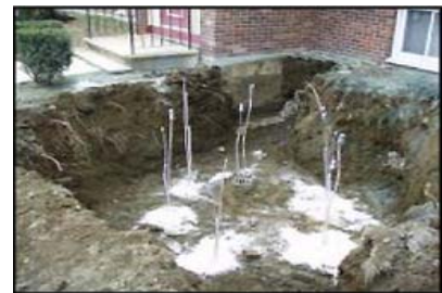
DX ground loop being installed at Claremont Arms Apartments. Six boreholes were drilled, with a copper U-loop tube in each. Tubes will be attached to supply and return headers, about 5 ft below grade, and inserted through the wall below the entry hall. White material is grout. [Photo by Mel Hensch.]
